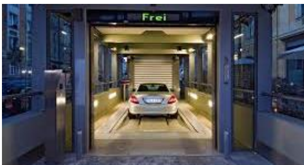
Figure 4. Receiving cabin in robotic car parking facility using car storage pallet
