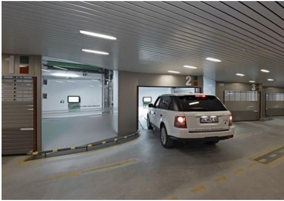
Figure 3. Entrance and exit of Robotic Parking Facilities [3]
